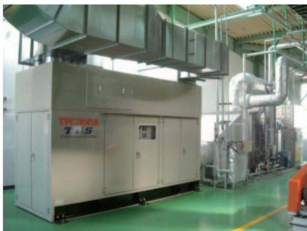
Fig. 2 Micro gas turbine Generation package Unit
